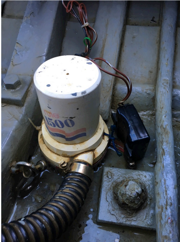
Bilge Pump and separate solid state 'float' switch.
