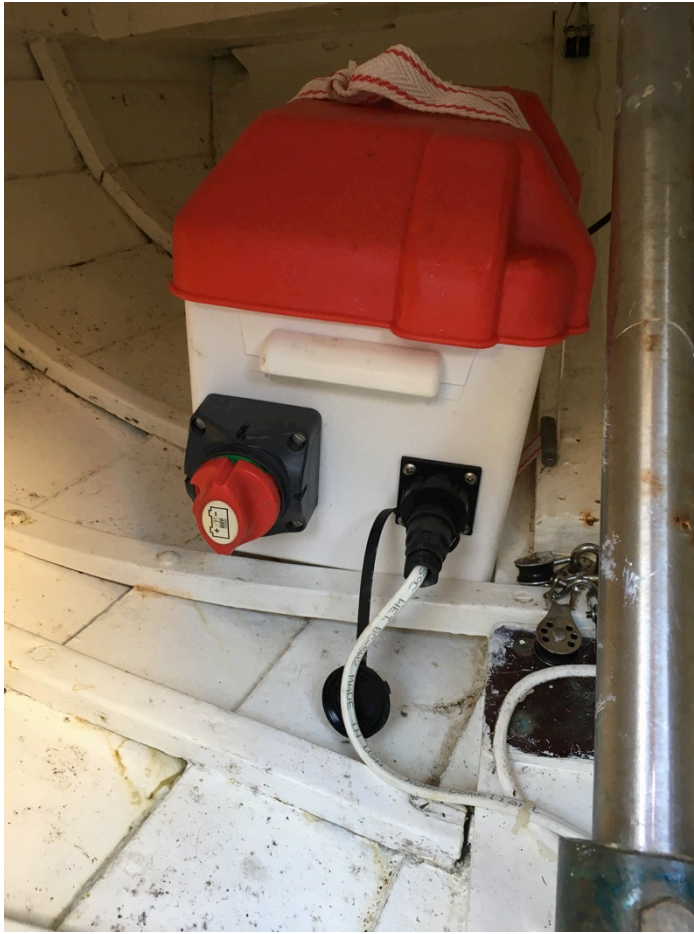
Self contained Battery Box solution as installed in aft locker
